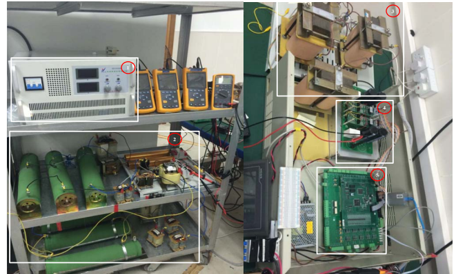
Fig. 12 Experimental Prototype (Note: ①-DC power supply; ②-Loads; ③-Coupling impedance; ④-IGBT and drivers; ⑤-Control board and signal conditional circuit.)
